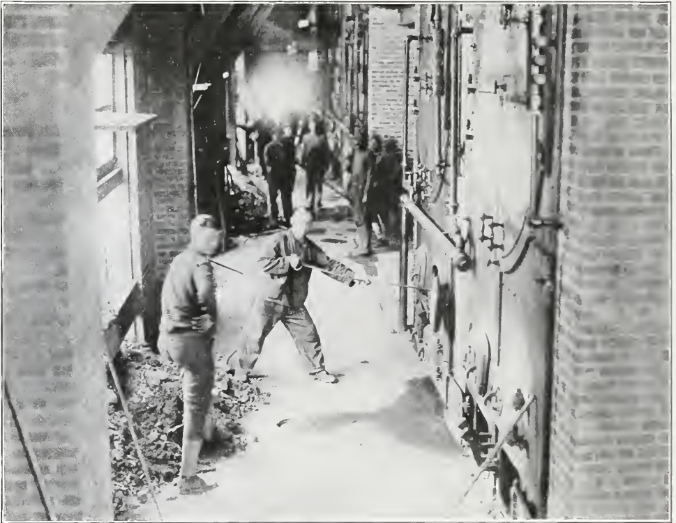
FIG. 161.—Interior of power and heating plant, Embarkation Hospital, Newport News, Va.
